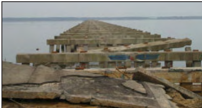
The bridge between Bay Saint Louis and Pass Christian was destroyed. Families and communities have been likewise disconnected. The enormity of this loss cannot be measured.
